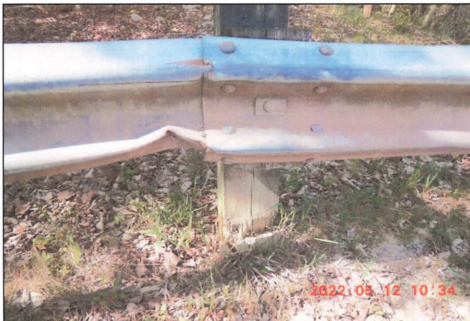
Photo 8: Fractured Post and Deformation on Southeast Approach Barrier
