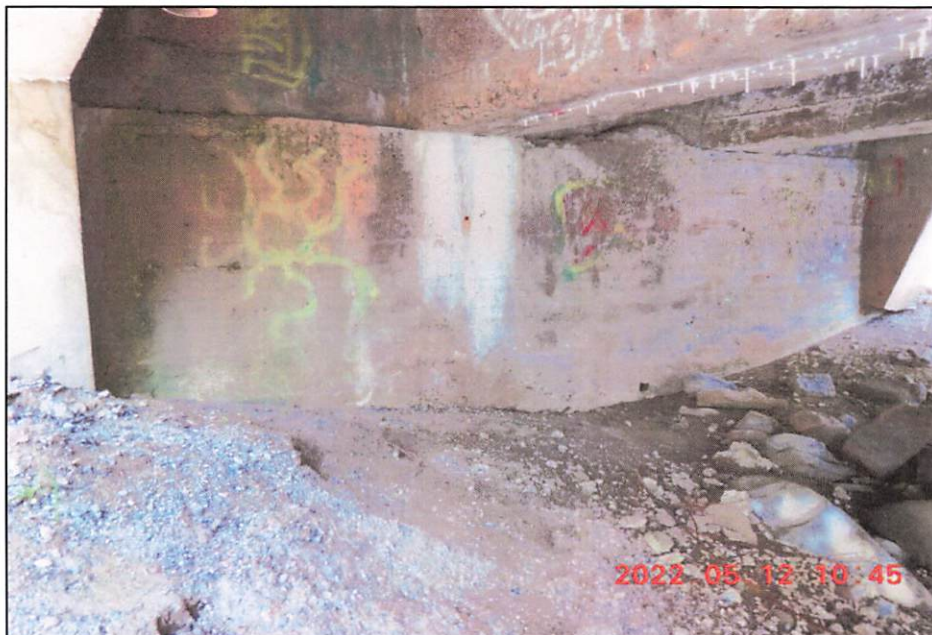
Photo 4: Efflorescence on West Abutment Wall and Scaling and Stalactites on T-Beam
