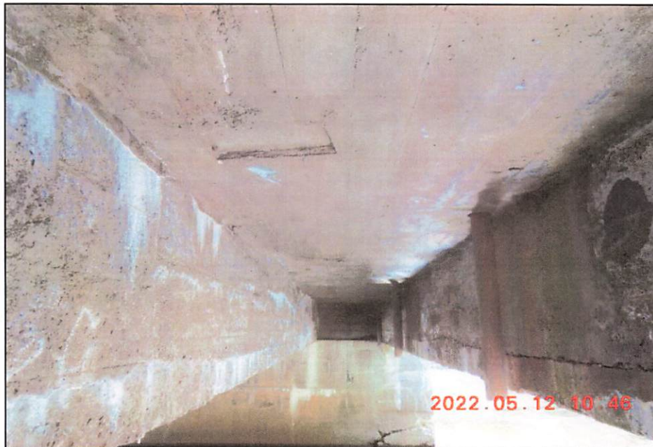
Photo 5: Cracking and Efflorescence on West Span Inter T-Beams and Soffit
