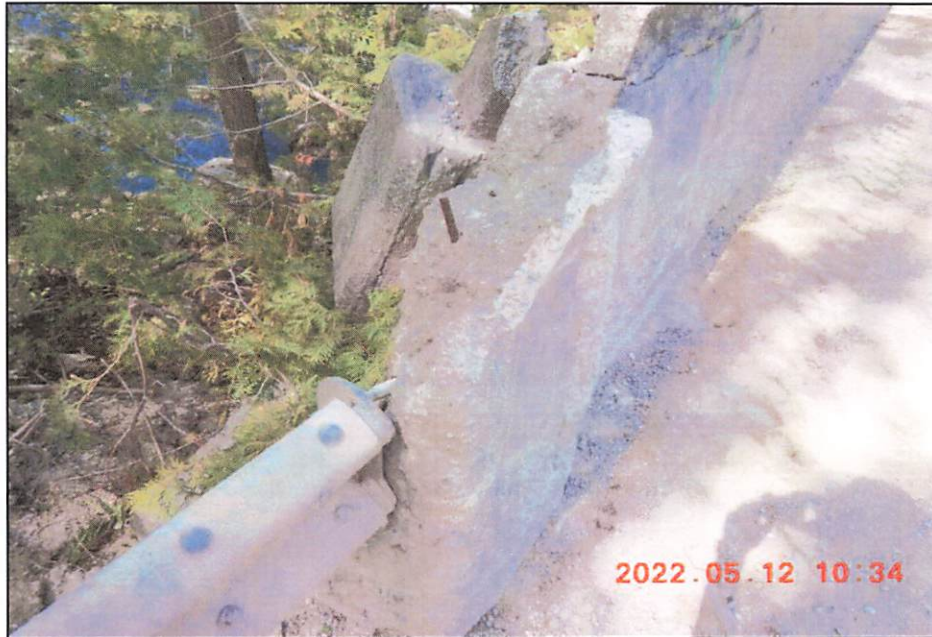
Photo 9: Spalling on Southeast Barrier Post
