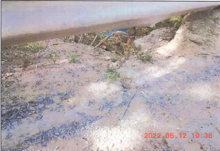
Photo 15: Erosion/Washout on Southeast Approach
