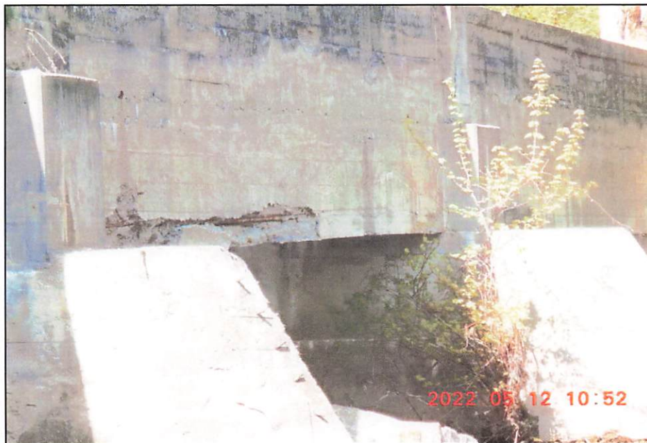
Photo 12: Spalling with Exposed Rebar on North Exterior T-Beam
