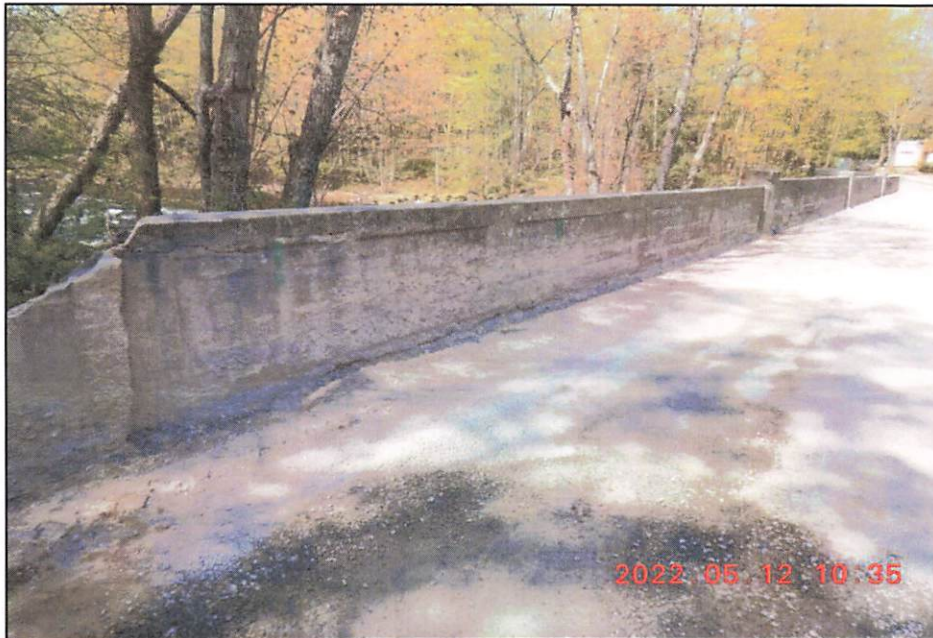
Photo 13: Scaling on South Interior Barrier Wall
