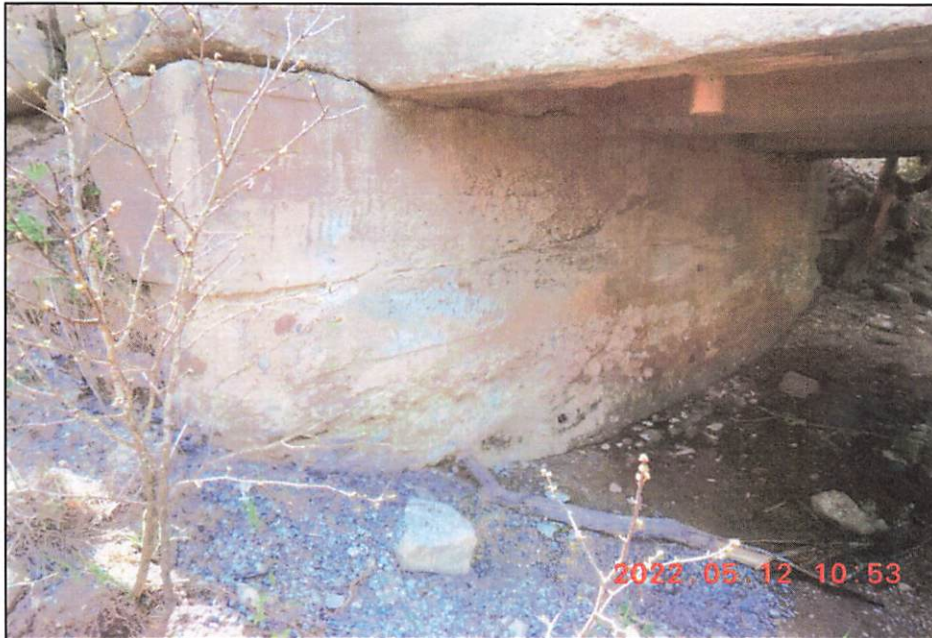
Photo 7: Erosion, Scaling and Cracking on East Abutment Wall
