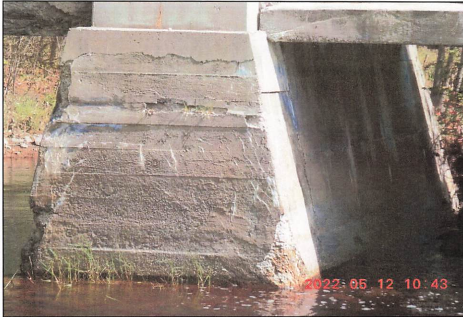
Photo 11: Scaling, Erosion, and Cracking with Efflorescence on West Pier South Face
